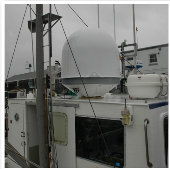
Satellite communications antenna on the roof of R/v Quest www.kvh.com
